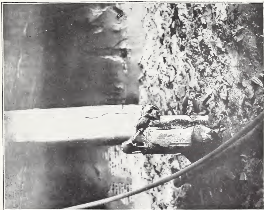
A. FAILURE OF BASEMENT COLUMN DUE TO FIRE, SLOANE BUILDING, SAN FRANCISCO.
